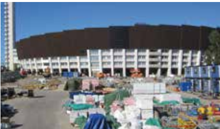
Helsinki Olympic Stadium with building site storage in front of the listed and renovated façade
